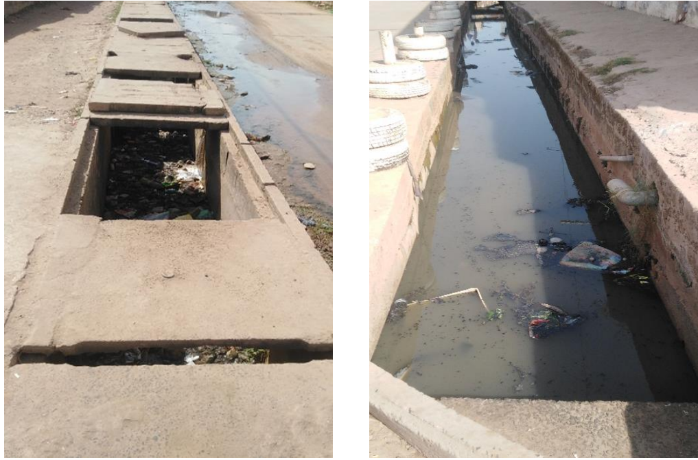
Figure 17. Inadequate Drainage System in Ebo Town
